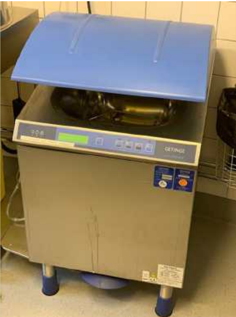
Figure 11-2: A closed bedpan washer at Sahlgrenska University Hospital, Sweden
