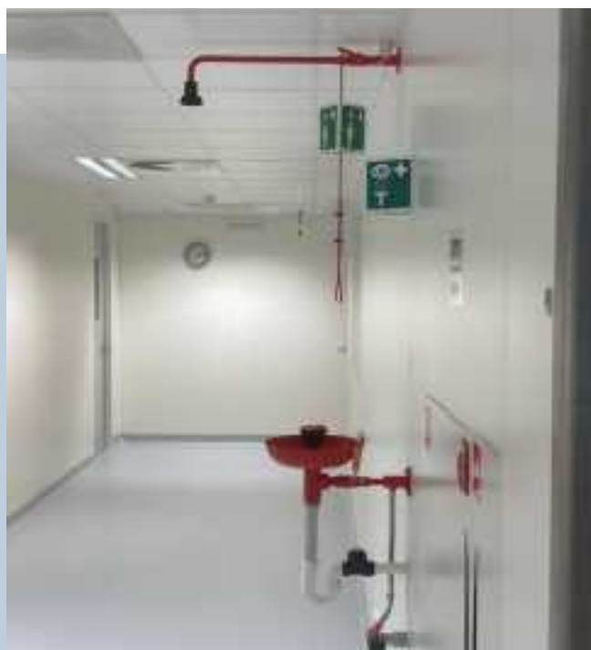
Figure 13-4: A shower and an eye shower in a pharmacy of a hospital (for emergency purposes in case of an incident) at the Meander Medical Centre, The Netherlands
